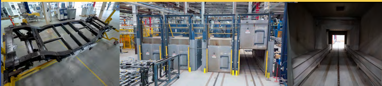
Curing Ovens & Paint Booths
