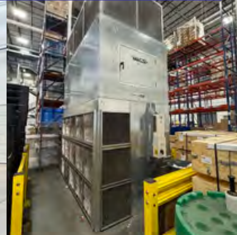
Industrial Air Systems
