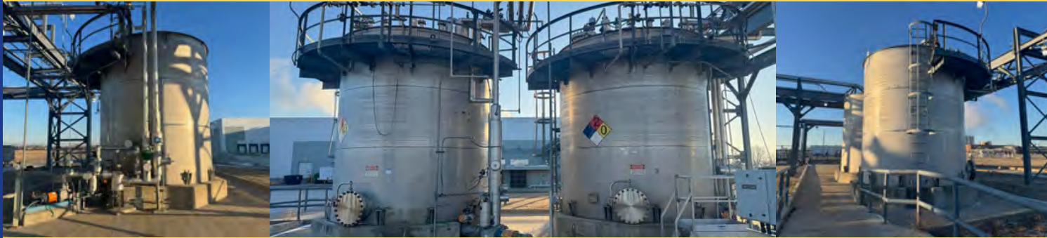
19,000-gallon storage vessel
