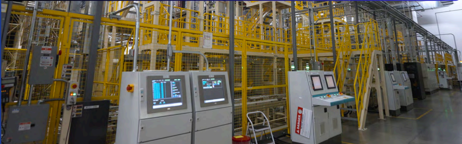
Multiple Muratec Automated Storage and Retrieval Systems, Kokam Casette Racking Systems
